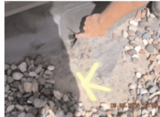
Visual Inspection Documents Typical Defective Conditions
